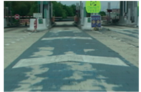
Epoxy markings after 1 year
