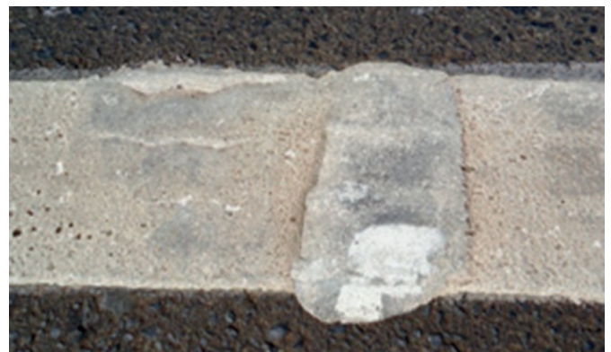
Profile marking based on thermoplastic road marking deformed within 1 year.
